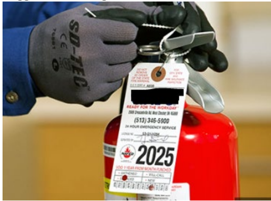
Tagged Fire Extinguisher
